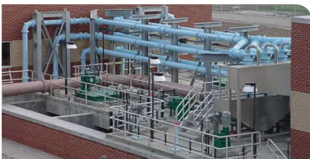
Lawrence, KS Lawrence wastewater treatment plant
